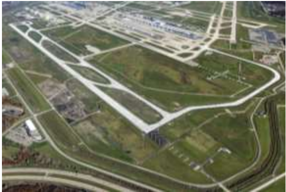
Detroit Metropolitan Wayne County Airport Reconstruction of Runway 4L and Associated Taxiways
